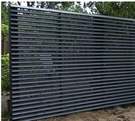
Img 27 - Painted horizontal timber
